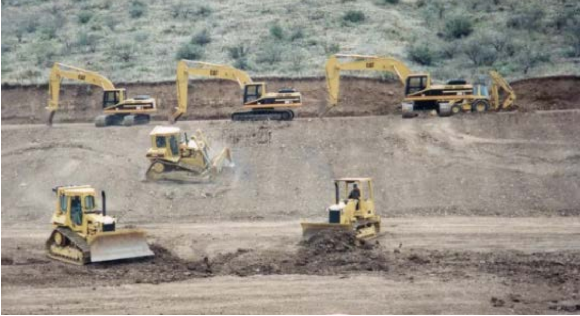
Figure 4. Clearing and Grading, the First Steps in Land Development. In Arizona and around the world, many patches of earth have succumbed to bulldozers, skidders, excavators, graders, and other heavy earth-moving equipment
